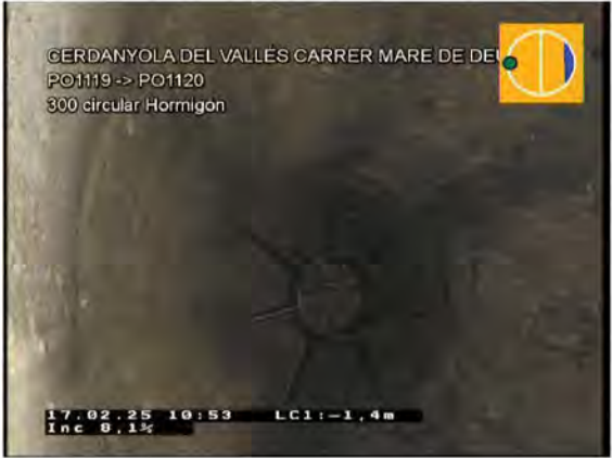
17_02_2025 10_00_01_4c3b9886-a4e4-4c88-9f24-9ce865e4442e_202502 17_105352_645.jpg, 00:02:44, 34.80m Nudo de final, registro,, PO1119
