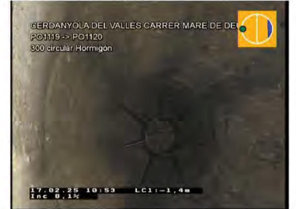
17_02_2025 10_00_01_4c3b9886-a4e4-4c88-9f24-9ce865e4442e_202502 17_105352_645.jpg, 00:02:44, 34.80m Nudo de final, registro,, PO1119
